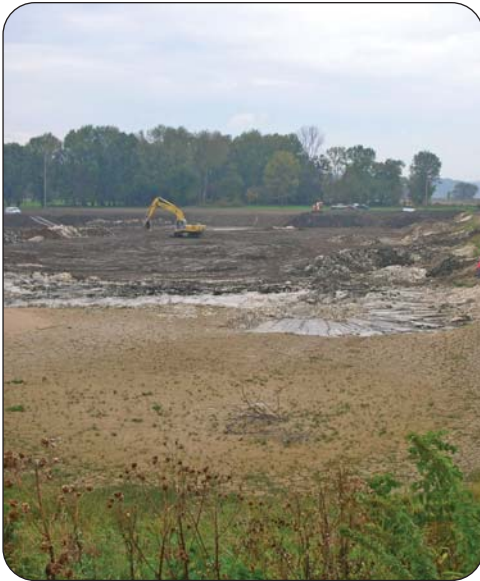
The City of Wooster Lime Lagoon Project.
